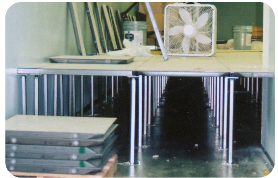
To allow room for an underfloor HVAC system, piping and computer wiring, Grunau's service and maintenance team oversaw the installation of a raised floor for Aurora Health Care's second computer room expansion.
