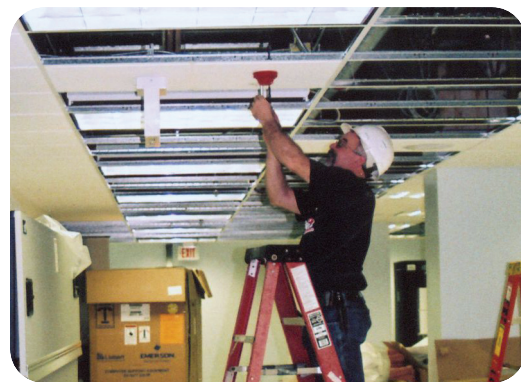
Grunau's fire protection and electrical teams installed a new fire suppression system in Aurora Health Care's second computer room expansion.
