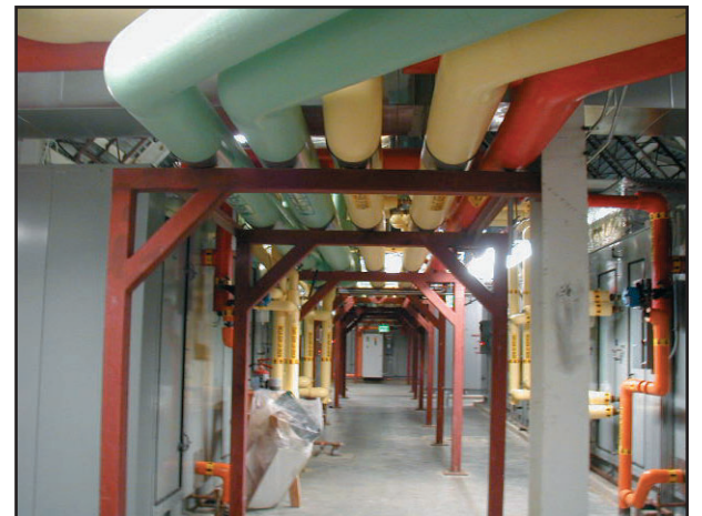
Grunau Fabricated Pipe Supports
