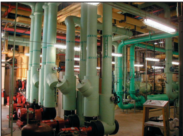
Chilled Water Pumps & Piping
