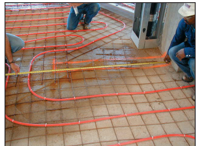
Lobby Underfloor Heating
