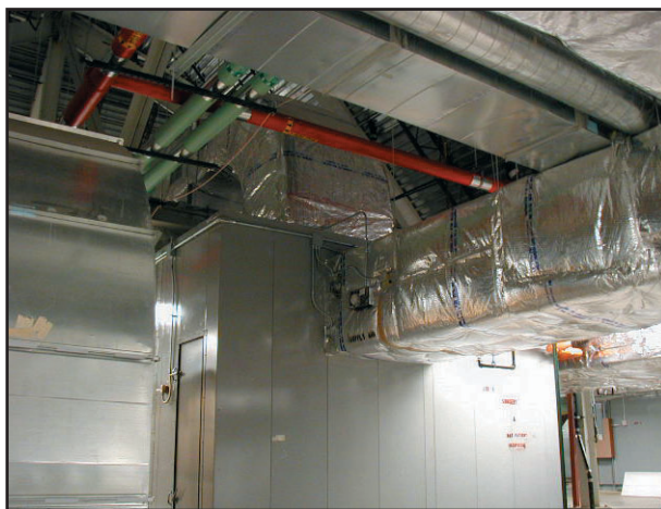
Mechanical Room Sheet Metal/Ductwork
