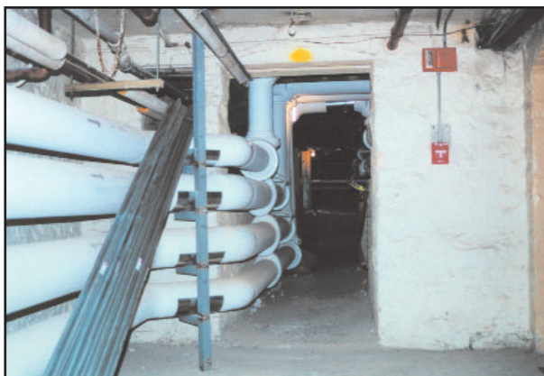
Typical Tunnel Piping
