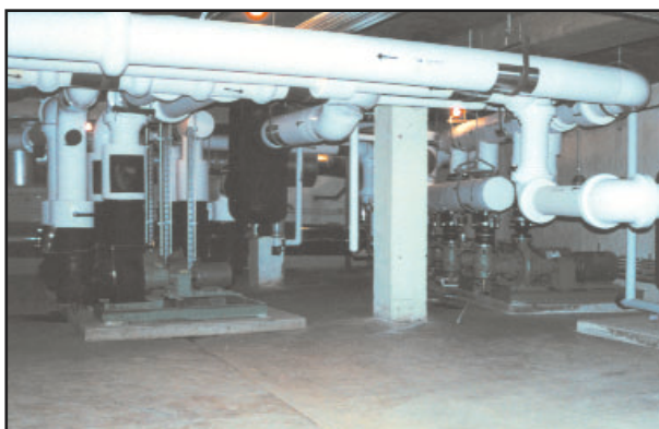
Main Pump Room
