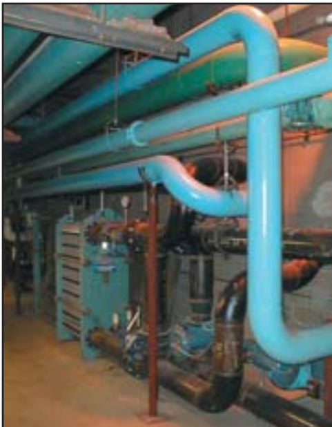
Reclaim Heat Exchanger & Piping
