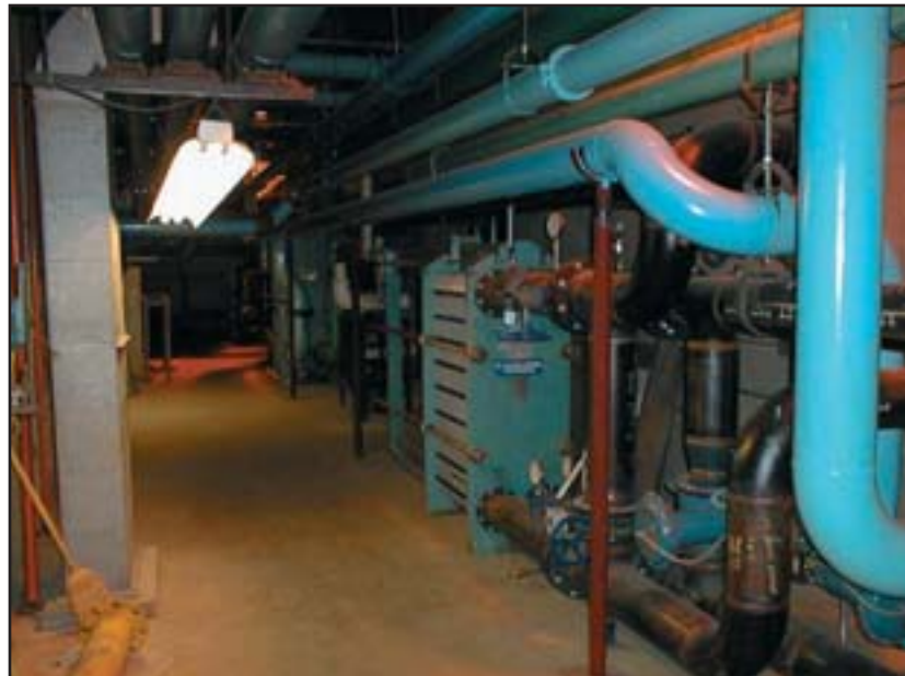
Heat Exchangers & Piping
