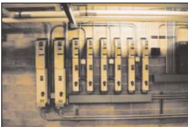
Variable Frequency Drives and Starters
