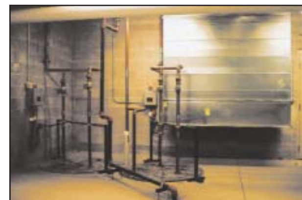
Duplex Pumps for Storm and Sanitary
