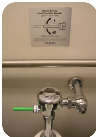
Grunau Company uses 50 percent less water than a typical office building thanks to new dual flush toilets.
