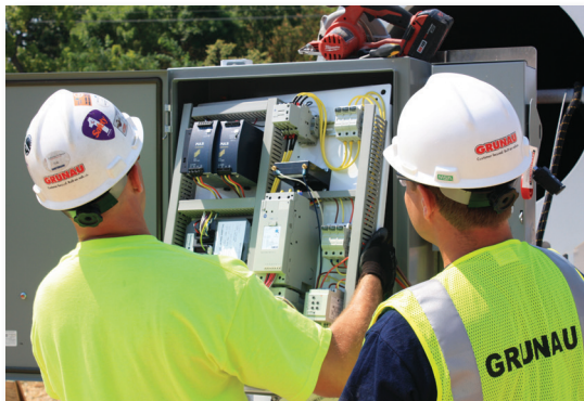
Electrical control panel at base of wind turbine
