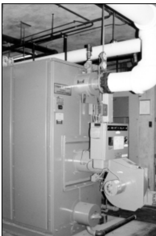
Hot Water Boilers
