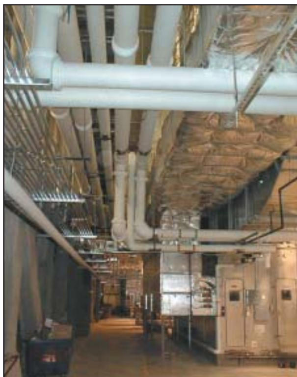
Mechanical Floor - Large Supply Air Plenum & Overhead Piping
