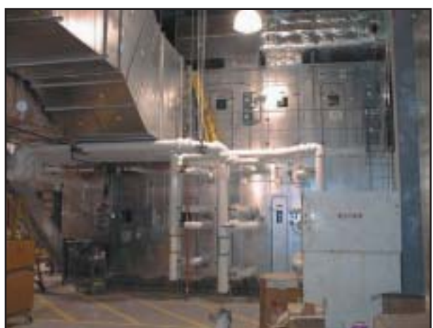
Mechanical Floor - Bi-Level Air Handling Unit
