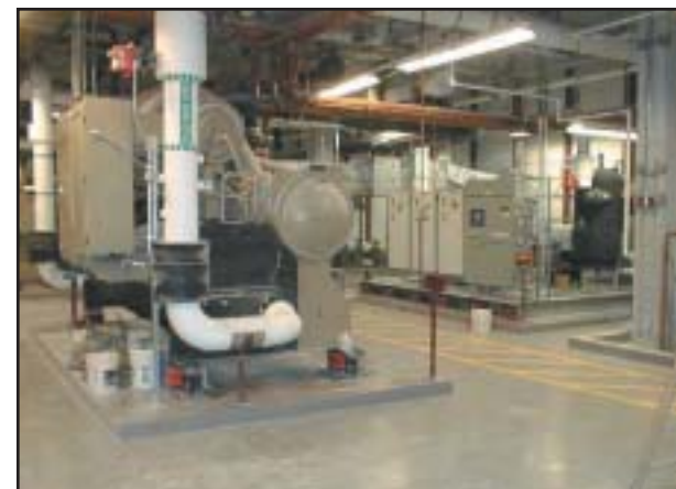
Penthouse Mechanical Room - Chiller
