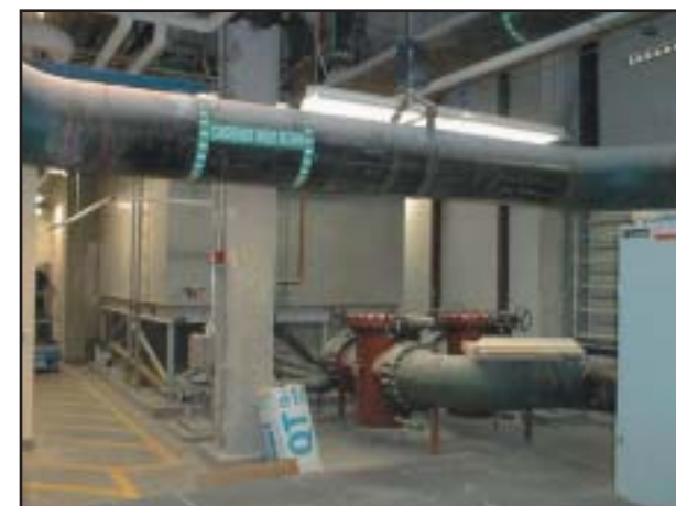
Penthouse - Remote Sump & Cond. Piping
